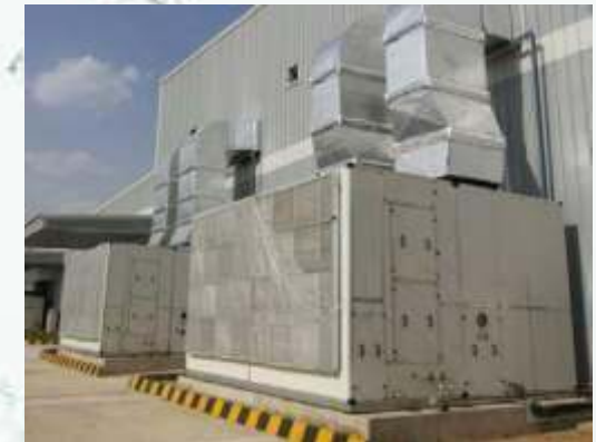
Air Cooling Units
